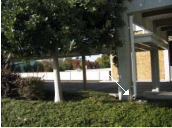
Rooftop runoff is directed to drain through the vegetation.
