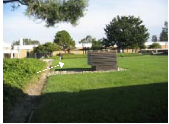
Exhaust vents for HVAC* systems are integrated into roof garden areas.
