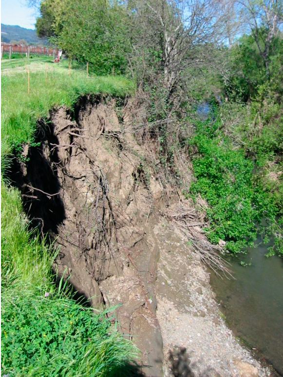
Photograph B-3. Bank collapse on Sequoia Grove property One of the priority restoration sites, this reach is stage 5, but receives impinging flows.
