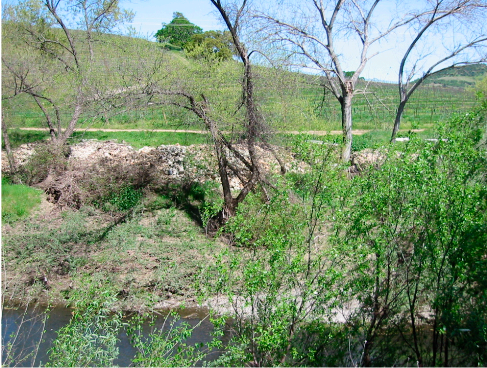
Photograph B-47. Rip rap protection on the Quintessa property, opposite mid point on Frogs Leap
