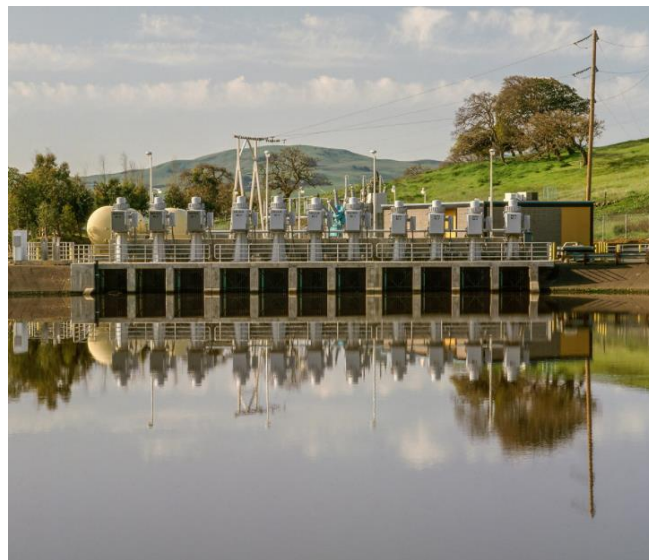
Figure 2-3. Cordelia Pumping Plant and Forebay
