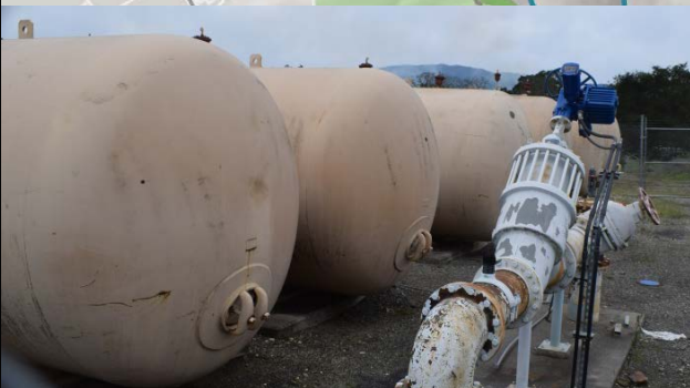
Yountville Treatment Plant
