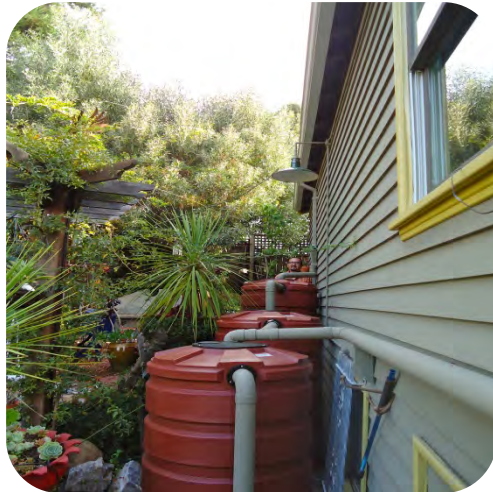
Daisy chained system of 205-gallon rain barrels Courtesy of The City of Oakland
